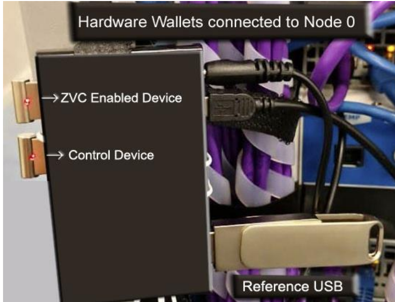
Mounted ZVC device & Control device
